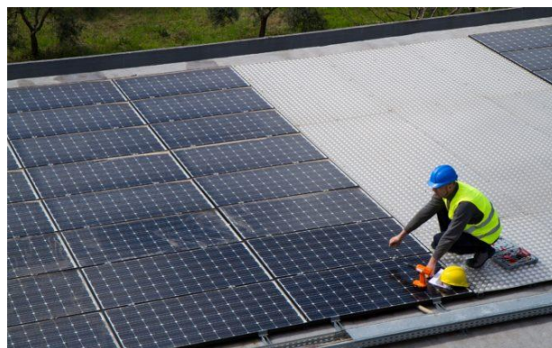
Figure 2 – Roof top solar
